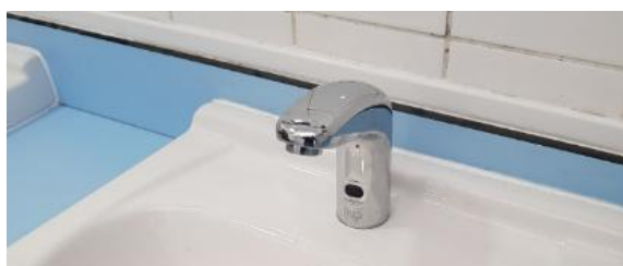
Figure 6: new hands-free taps, with on demand heating, installed at Palace Green toilets, Ely
