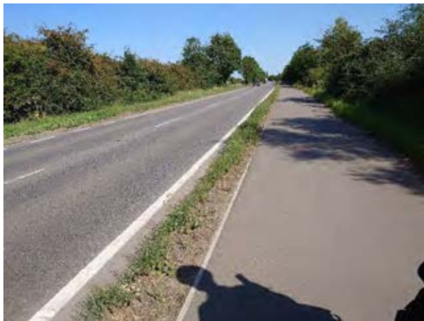
Figure 7C 7.1 The existing segregation from high speed traffic is inadequate.
