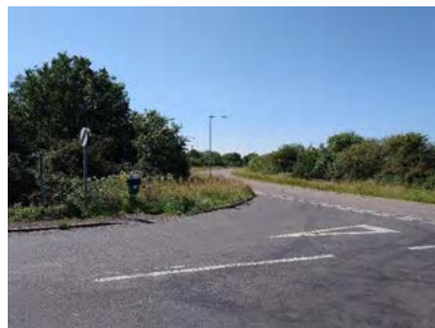
Figure 7B 2.1 showing the wide junction at the entrance to the closed road. This needs amending – see Option A.
