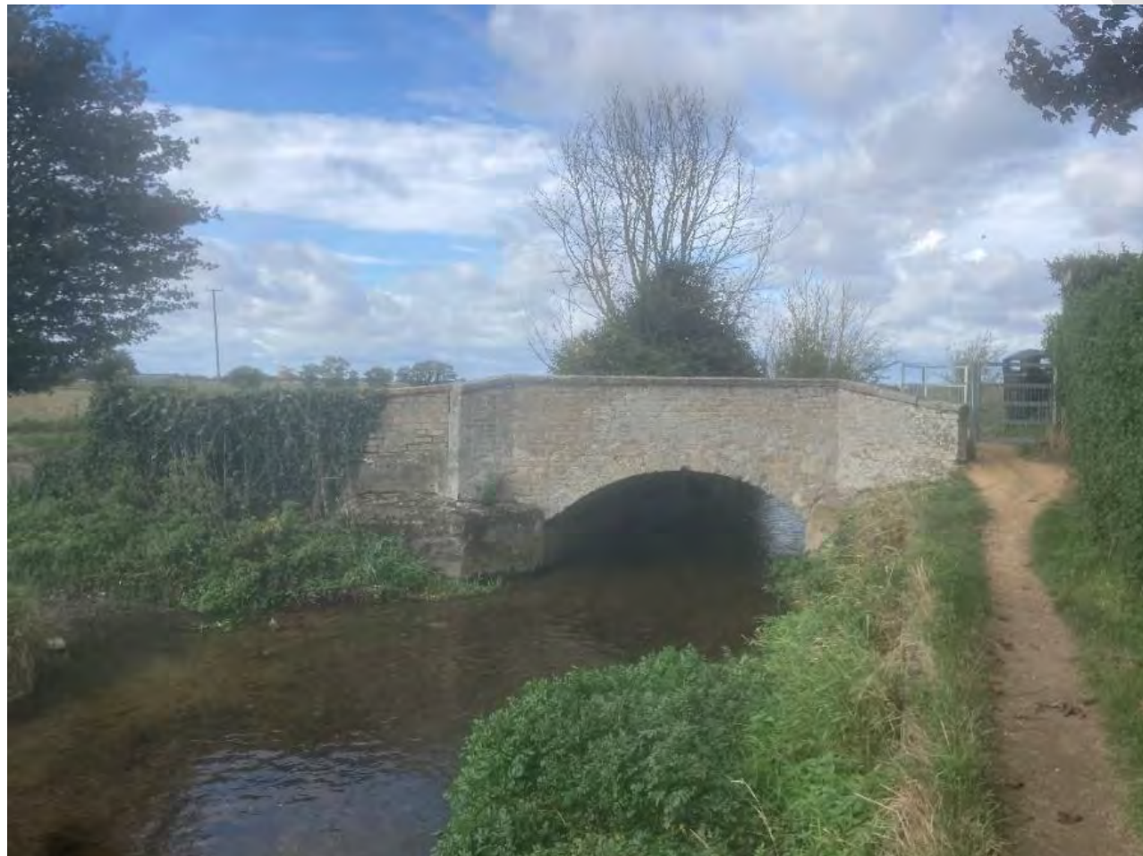
Figure 6.6.1 – River Snail bridge and associated access issues.
