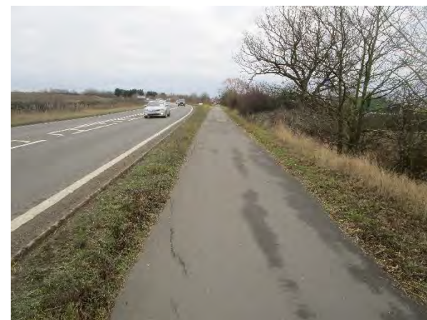
View of existing A142 path , which makes maximum use of the limited verge space, but does not comply with the spacing required in LTN 1/20.
