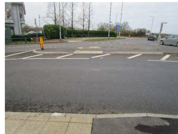
The existing crossing does not comply with current recommendations. It needs to be reduced to a single lane with a parallel crossing suggested. Kerbs need realigning. Detailed design is needed.
