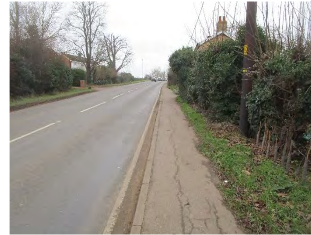
West End in Wilburton by start of footpath. Not suitable to promote as a cycle route for inexperienced riders.
