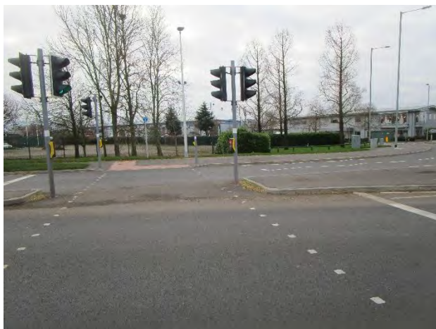
The existing crossing does not comply with current recommendations, but changing it at this moment is low priority.
