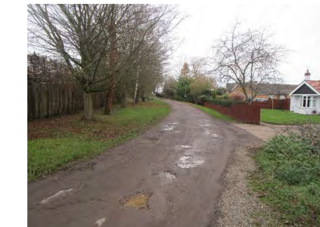
Hinton Way needs resurfacing to the junction with Clarke's Lane.
