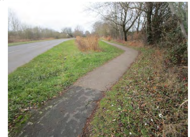
This path needs widening to 3m and to be designated as cycling only. Careful design to protect ecology is needed.
