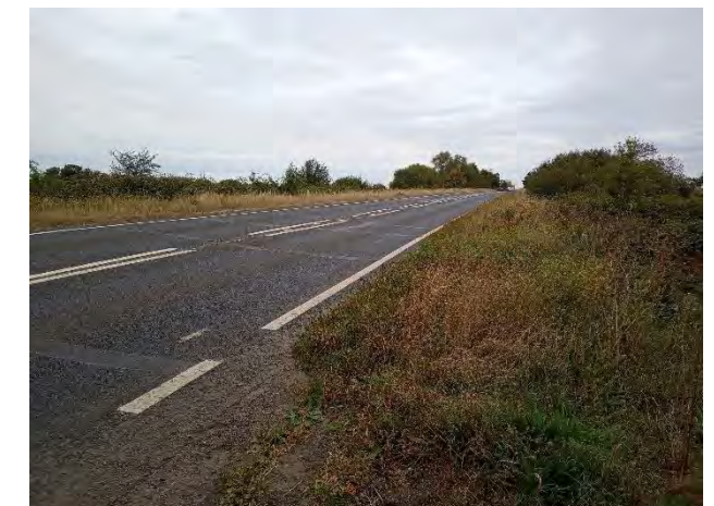
Figure 7.1.10.3 View of the existing A10 verge where a path would need to be built that is adequately separated from the busy road.
