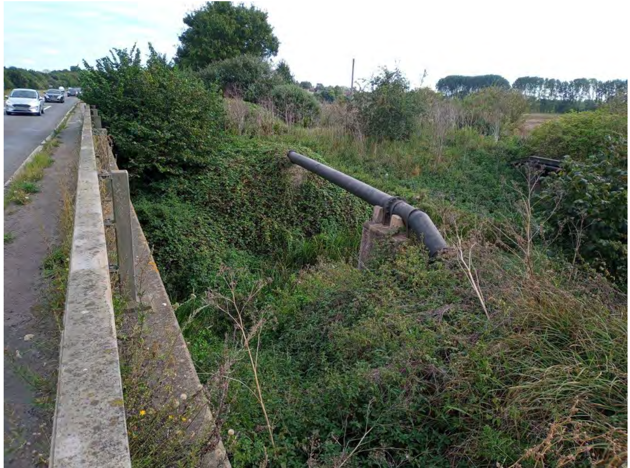
Fig 6.7 showing existing main water pipe found along proposed route alignment A and C
