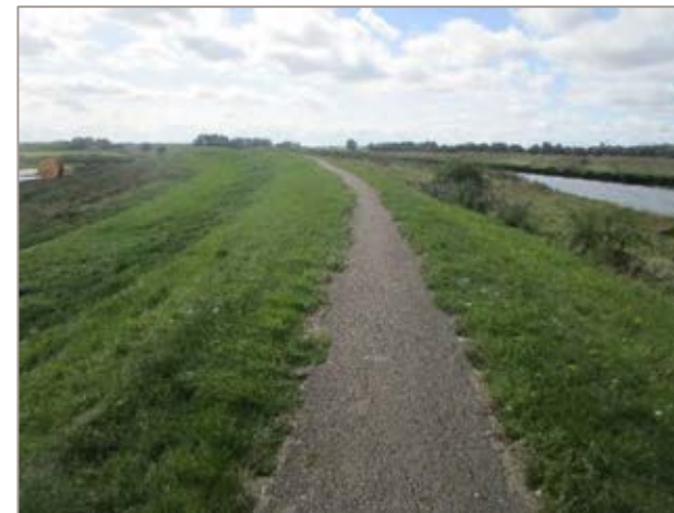
Figure 7D.8.2 showing flood bank with foot of flood bank and field edge.
