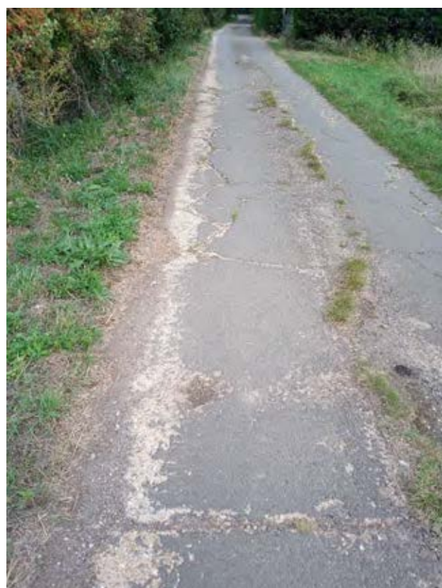
Fig 7C.13.1 Nornea Lane showing cracking and uneven surface.
