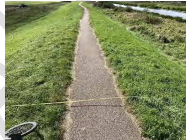
Figure 7D.8.1 showing flood bank with narrow path and tape indicating 3m width.
