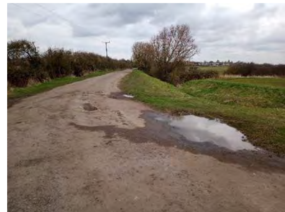
Pothole repairs and some resurfacing is needed on Hurst Lane.
