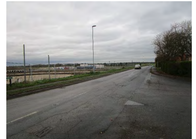
View along Newmarket Road towards disused railway showing development works underway (December 2021)
