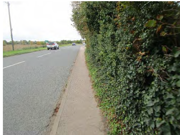
Existing shared use path besides Fordham Road. This feels very unsafe, especially with fast traffic on the road.
