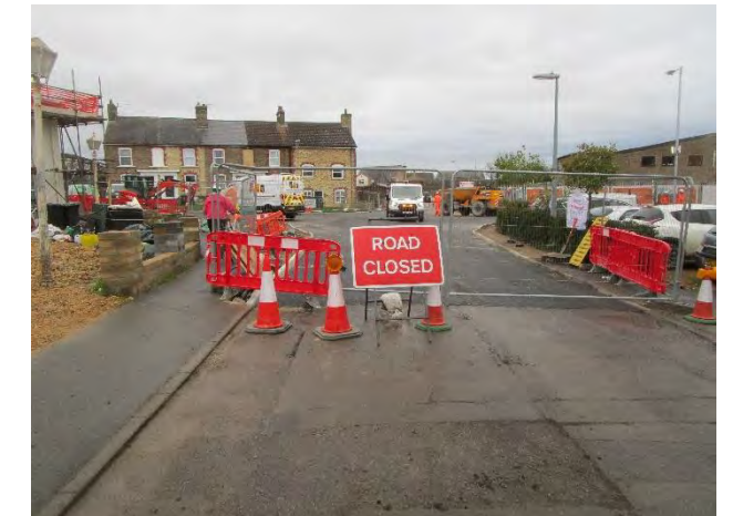
At the time of survey roads around the new station were closed to through traffic and the town was continuing to function.
