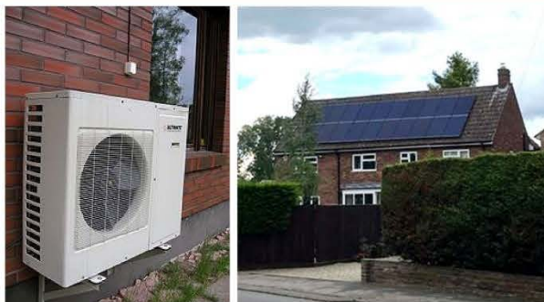
Ground/air source heat pump and solar panels
