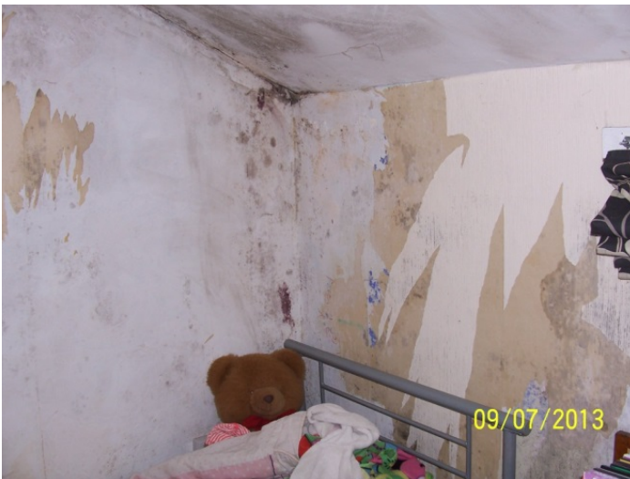
Figure 6: Hazard of damp and mould growth in East Cambridgeshire
