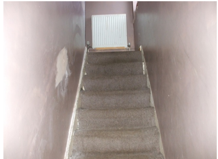
Figure 5: A missing balustrade presenting a falling on stairs hazard in East Cambridgeshire
