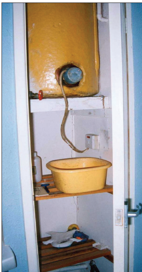
Airing cupboard with hot water tank above
